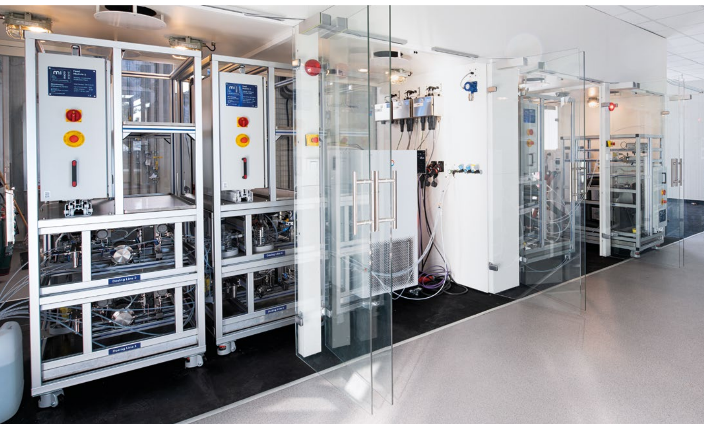
Flow chemistry manufacturing facility at CordenPharma Chenôve (FR)
