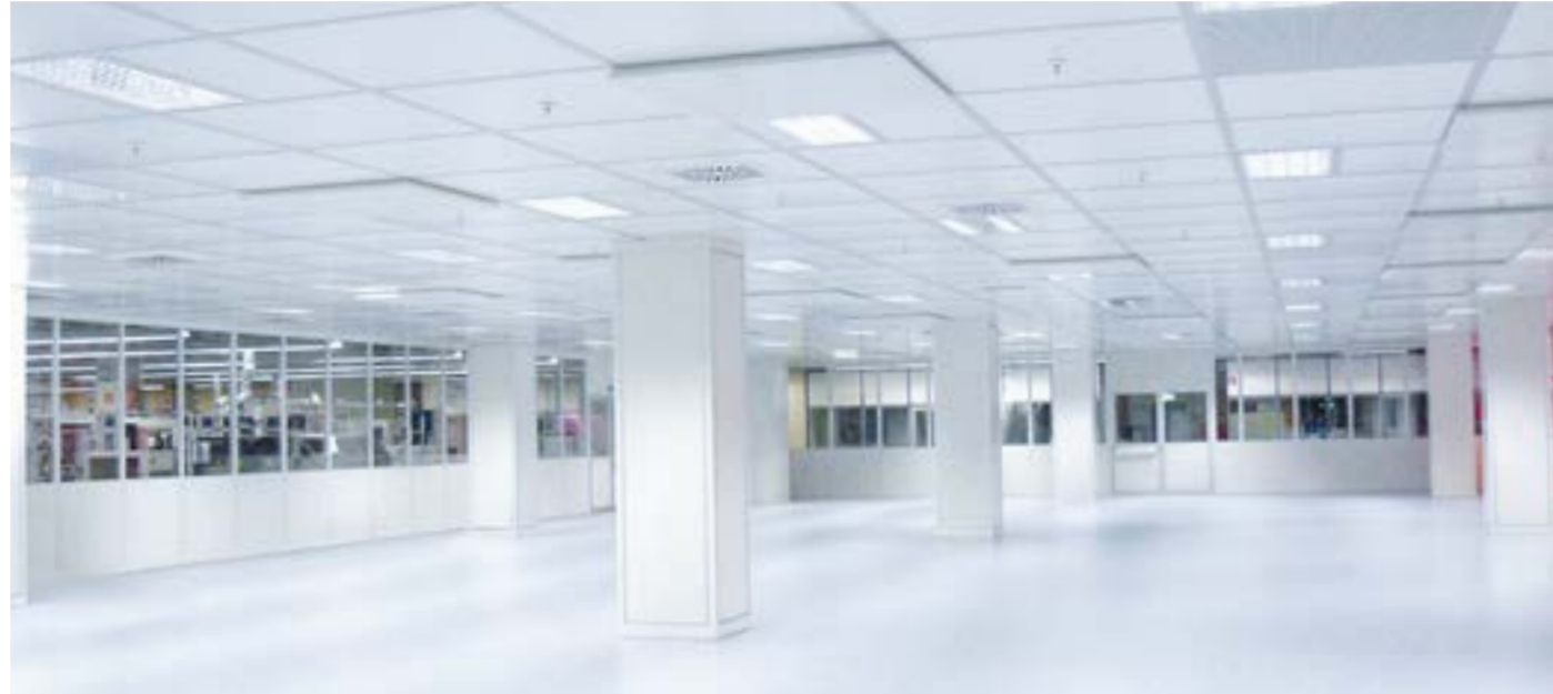
Cleanroom solutions according to VDI, ISO, GxP and controlled rooms according to VDA 19
