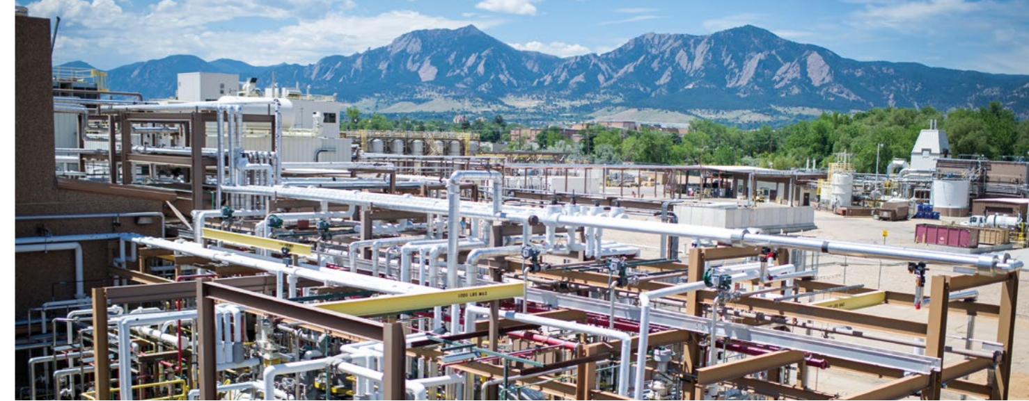
View of our Highly Potent & Oncology facility CordenPharma Colorado (USA).
